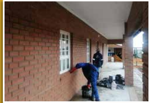
Final stage on the construction of a classroom block at Tharollo Primary School.
