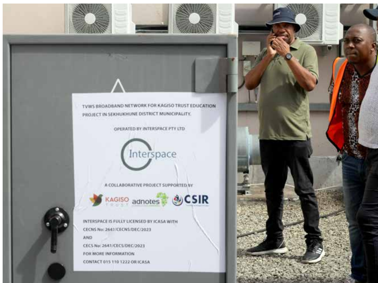
Site visit to the TVWS tower in Thaba Moshate at Burgersfort.
